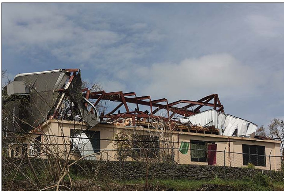
DESTRUCTION: Damage from Cyclone Pam in Port Vila in March 2015. Copyright International SOS, 2015.
